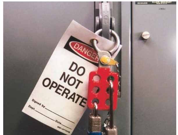
FIGURE S-5 The equipment can be locked out by several different people.
